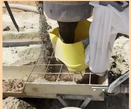
Ranger’s sample waste chute was designed in-house with significant input from field crews to ensure a practical solution that reduced risk of injury.
